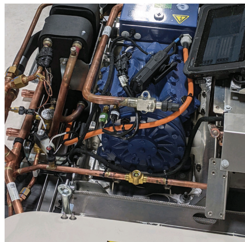
Roof-Mounted Electric HVAC
